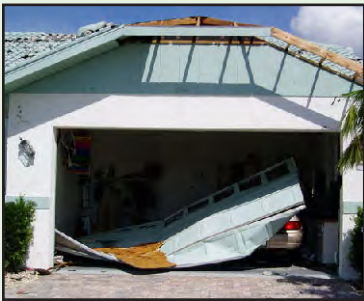
Figure 4-12: Because of their width, double-wide garage doors are more susceptible to wind damage than single doors. 19 (Source: Florida Hurricane Depot)
