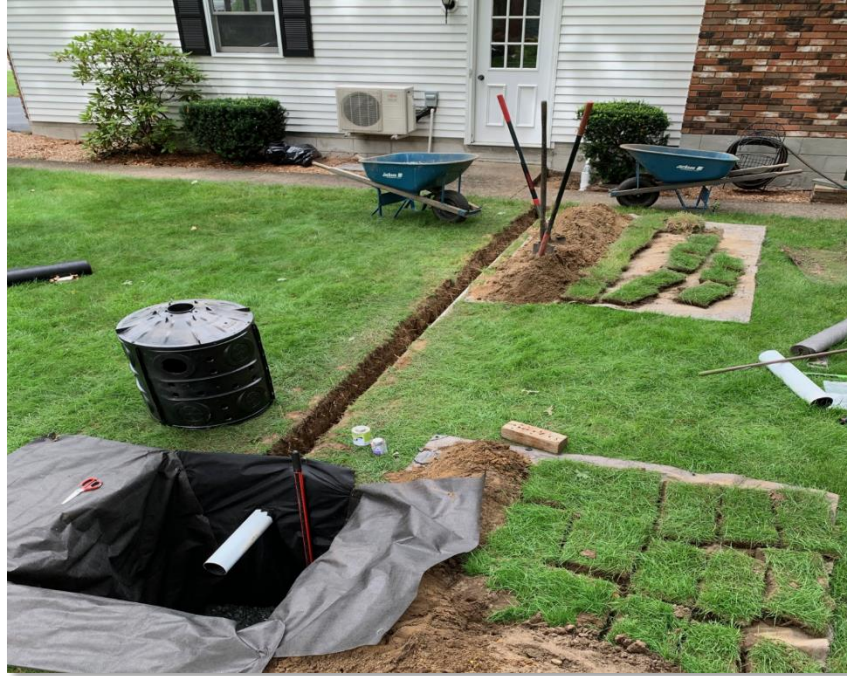
Image 1: New sewer lateral (white pipe) being installed between residence and new grinder package (black structure)
