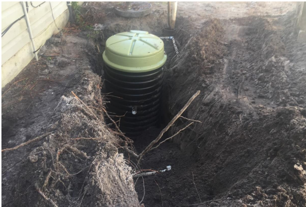
Image 2: New grinder package (black structure with green cover) being installed adjacent to existing structure.
