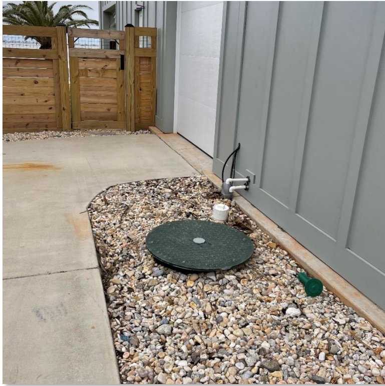
Image 3: Grinder package after installation is complete. Only the access cover is visible from the surface.
